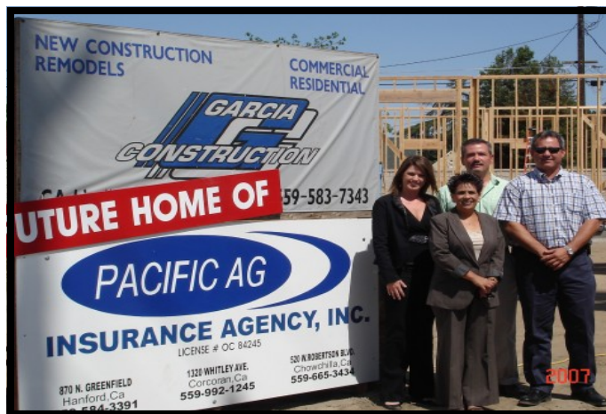
Standing near the new building site are left to right, Kristen Morton, Don and Jimmy Heskett and Georgina Garza in front.
